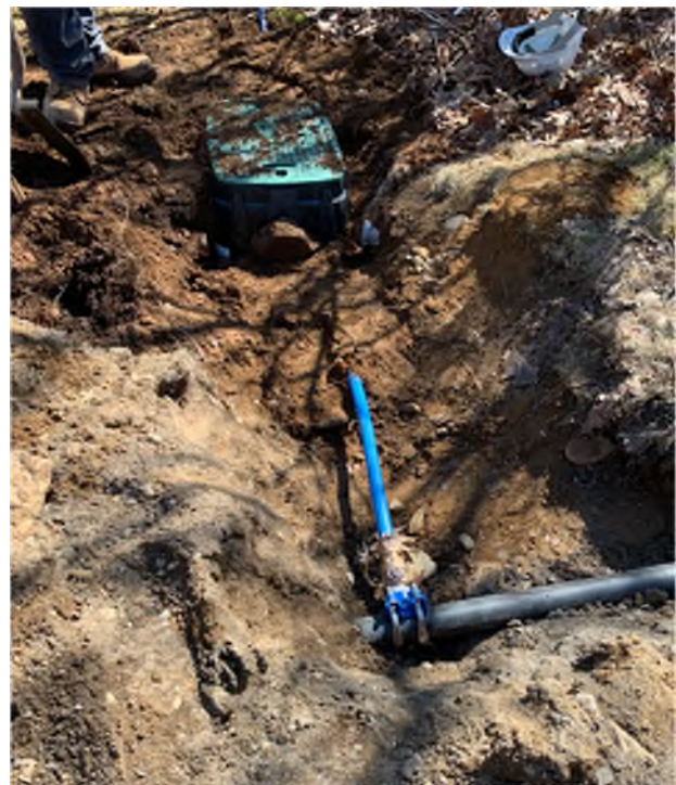
1" HDPE Seasonal Service Connection
