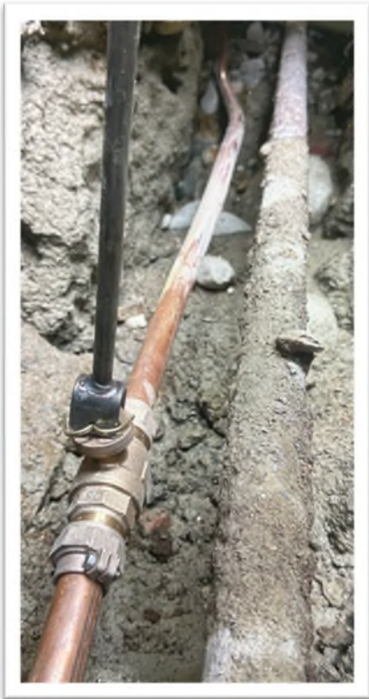
Replaced the last known lead service line in Portland, pictured to the right, with a new copper pipe, pictured to the left.
