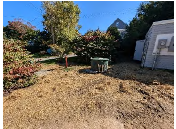
Ottawa Road Pump Station – Installed in 1976 – in the process of being upgraded
