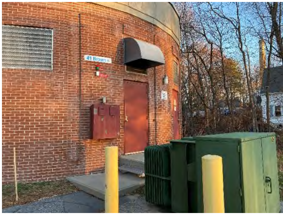
Cottage Street Pump Station
