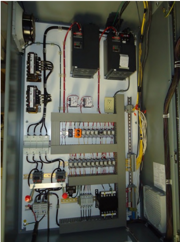
The SCADA panel for the newly installed Great Pond Pump Station for the Peaks Island Sewer Extension Project
