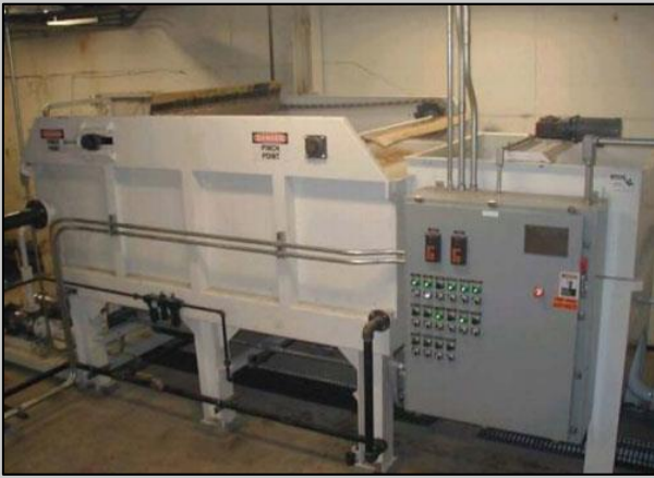
Worked with Schlotterbeck and Foss to upgrade their pretreatment system by installing a Dissolved Air Flotation(DAF) unit.
