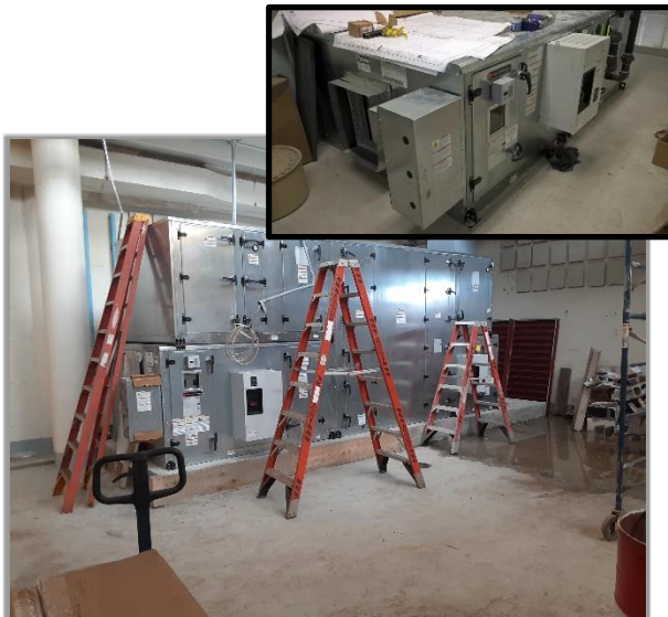
Manage construction phase of EEWTF Dewatering Area and CEWWTF Headworks HVAC upgrades.
