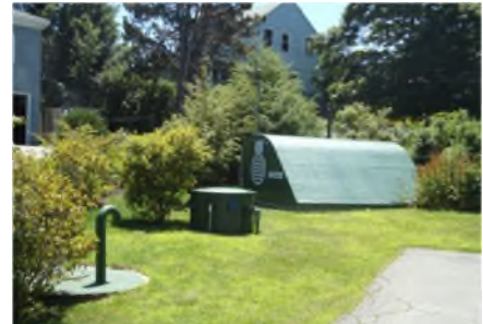
Ottawa Road Pump Station – Installed in 1976 – scheduled for upgrade in 2021
