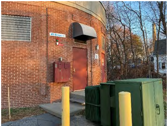
Cottage Street Pump Station
