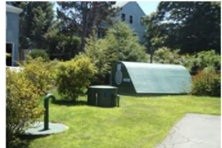
Ottawa Road Pump Station – Installed in 1976 – in the process of being upgraded
