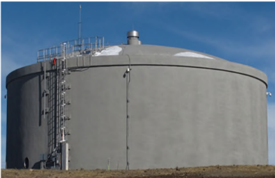
Managed and supported Windham Storage tank replacement project – water main installation and initiation of tank construction
