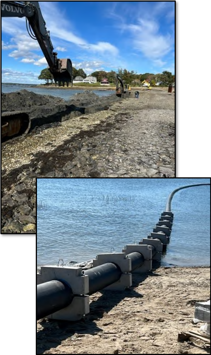
Managed design and construction of twin submarine main replacement between Great and Little Diamond Islands
