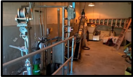
New Peaks Island Treatment Facility's Influent Screen Rotated out of the Channel for Inspection
