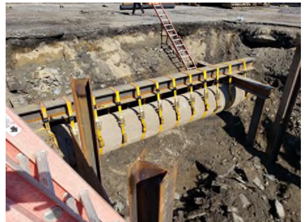
Pictured: India Street 33” pre-stressed Force Main exposed during installation of City Storm Sewer in 2019
