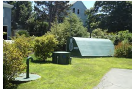
Ottawa Road Pump Station – Installed in 1976 – in the process of being upgraded
