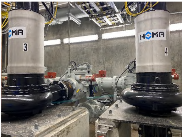
Dana Court Pump Station New dry pit submersible pumps installed in 2019
