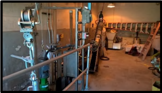
New Peaks Island Treatment Facility's Influent Screen Rotated out of the Channel for Inspection
