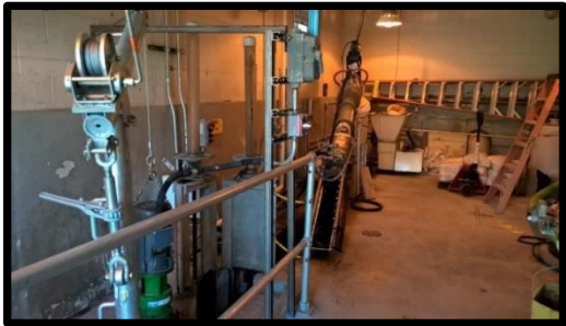
New Peaks Island Treatment Plant's Influent Screen Rotated out of the Channel for Inspection
