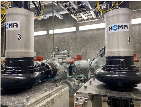
Dana Court Pump Station New dry pit submersible pumps installed in 2019
