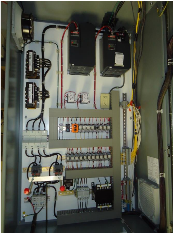
The SCADA panel for the newly installed Great Pond Pump Station for the Peaks Island Sewer Extension Project
